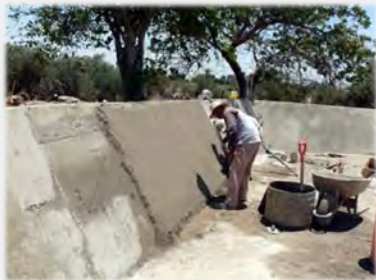
Some of the repairs that needed to be done to the camp pool in Betel as a result of the 2007 earthquake.
